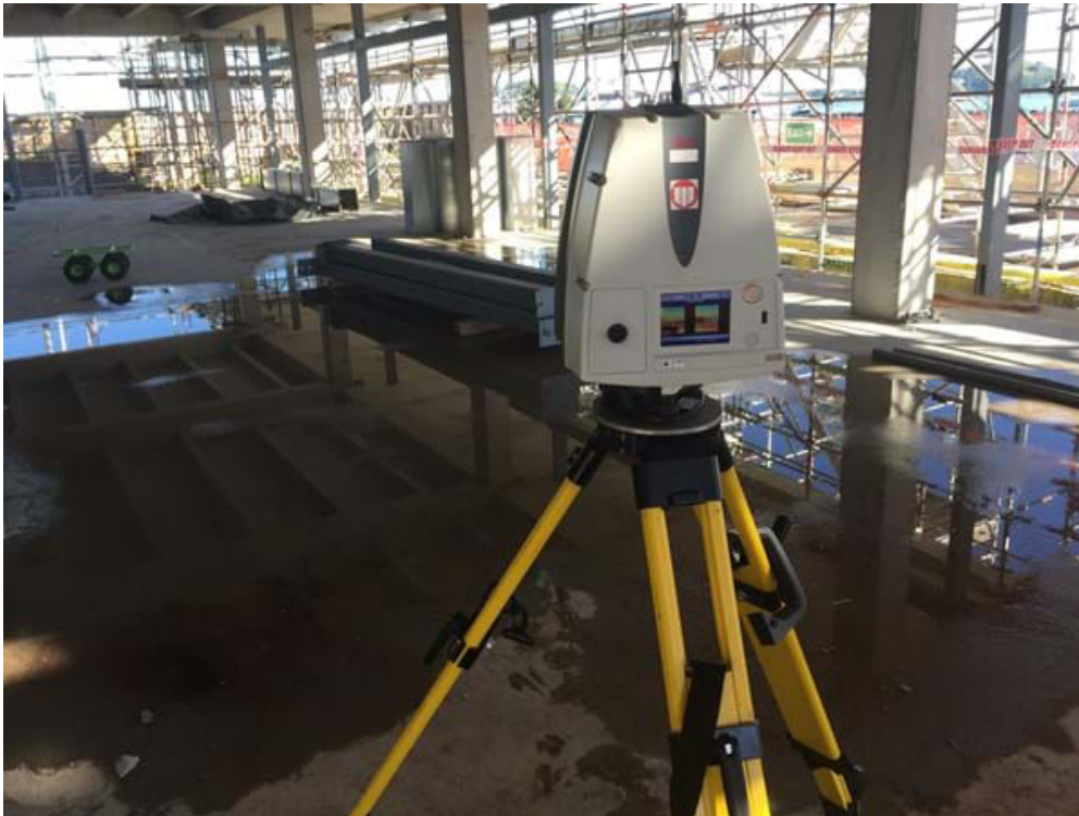
Leica Scan Station P-series 3D laser scanner
